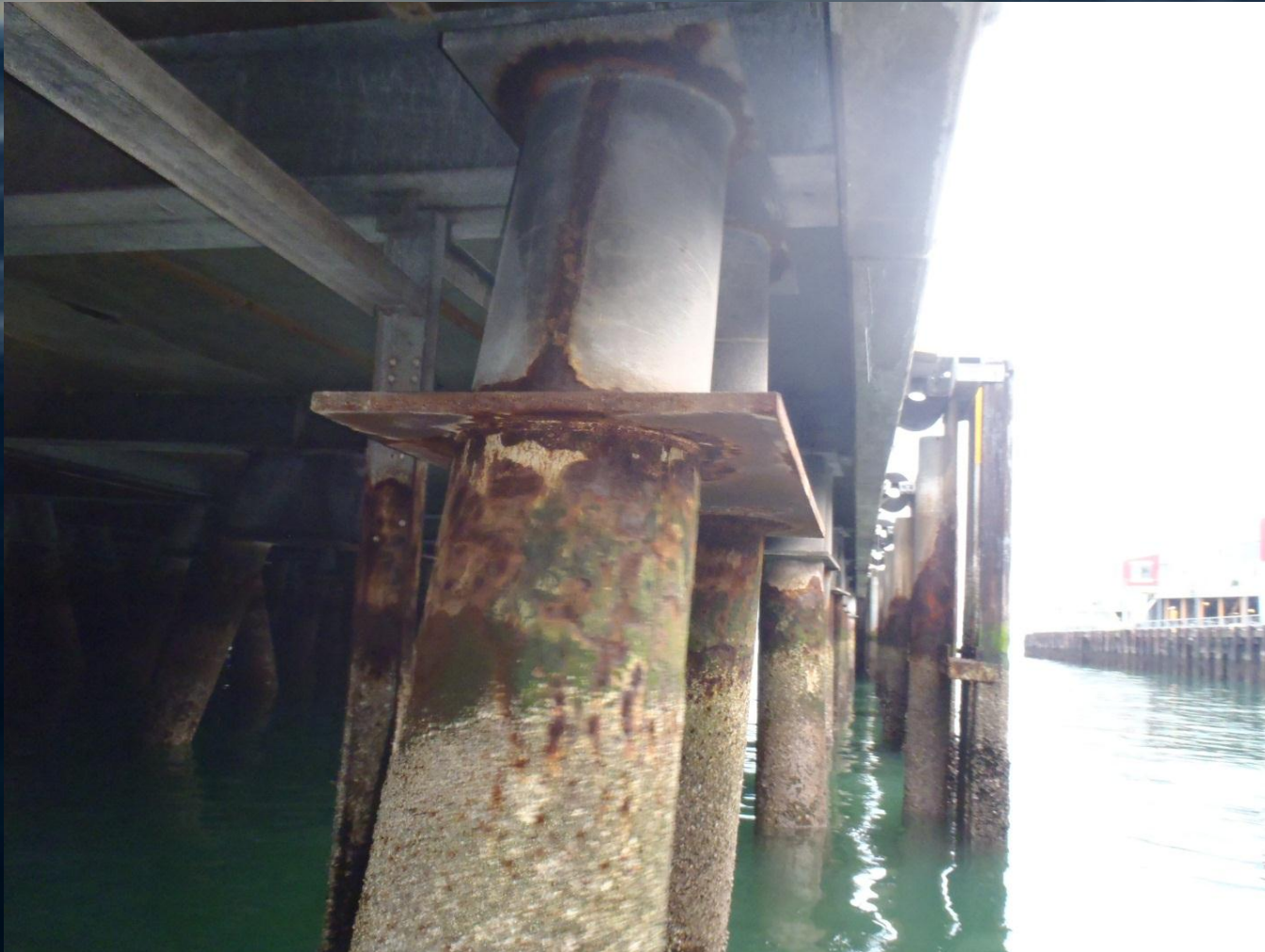
PILING CORROSION, PIER 69
