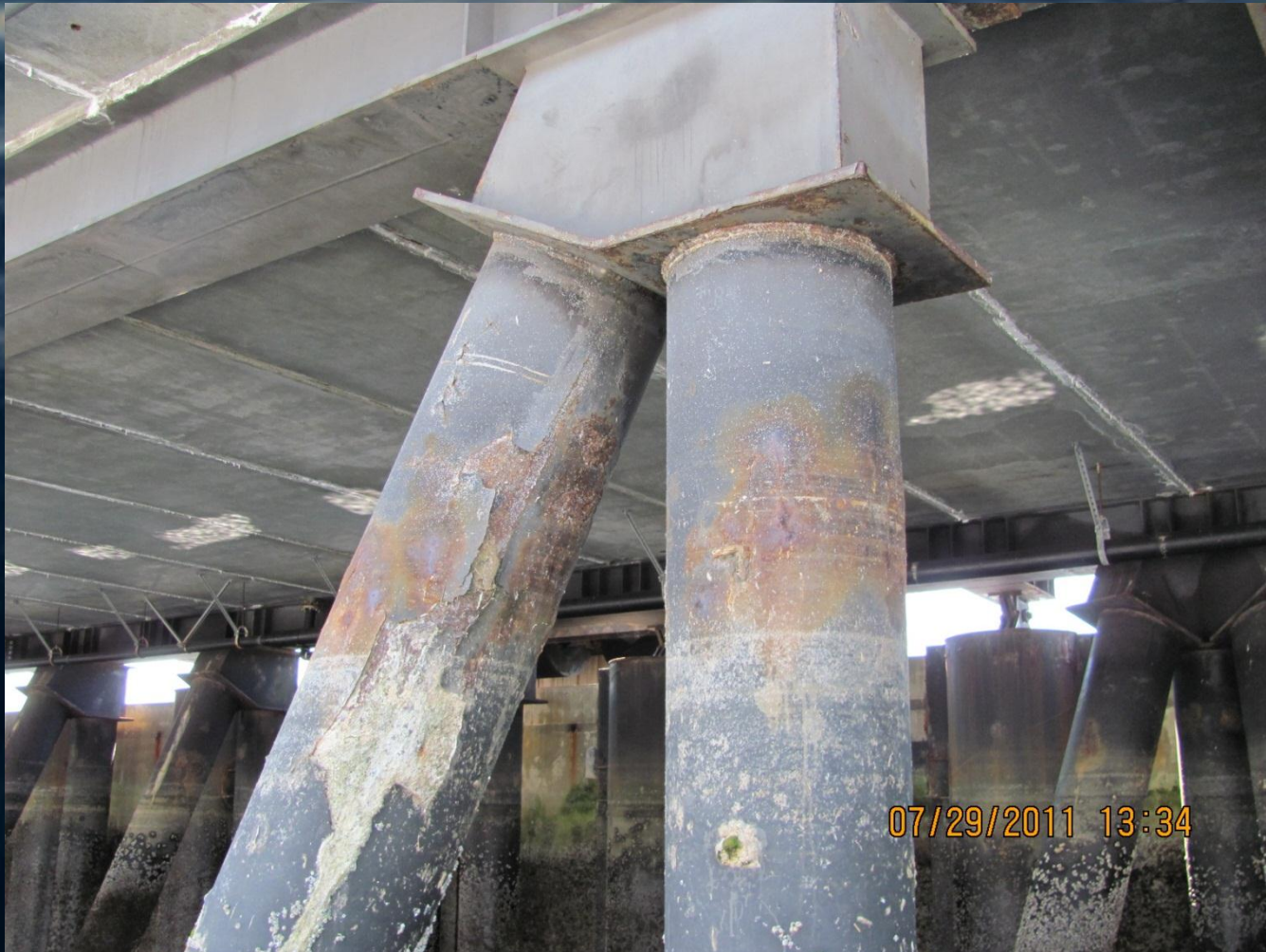
PILING CORROSION, PIER 66
